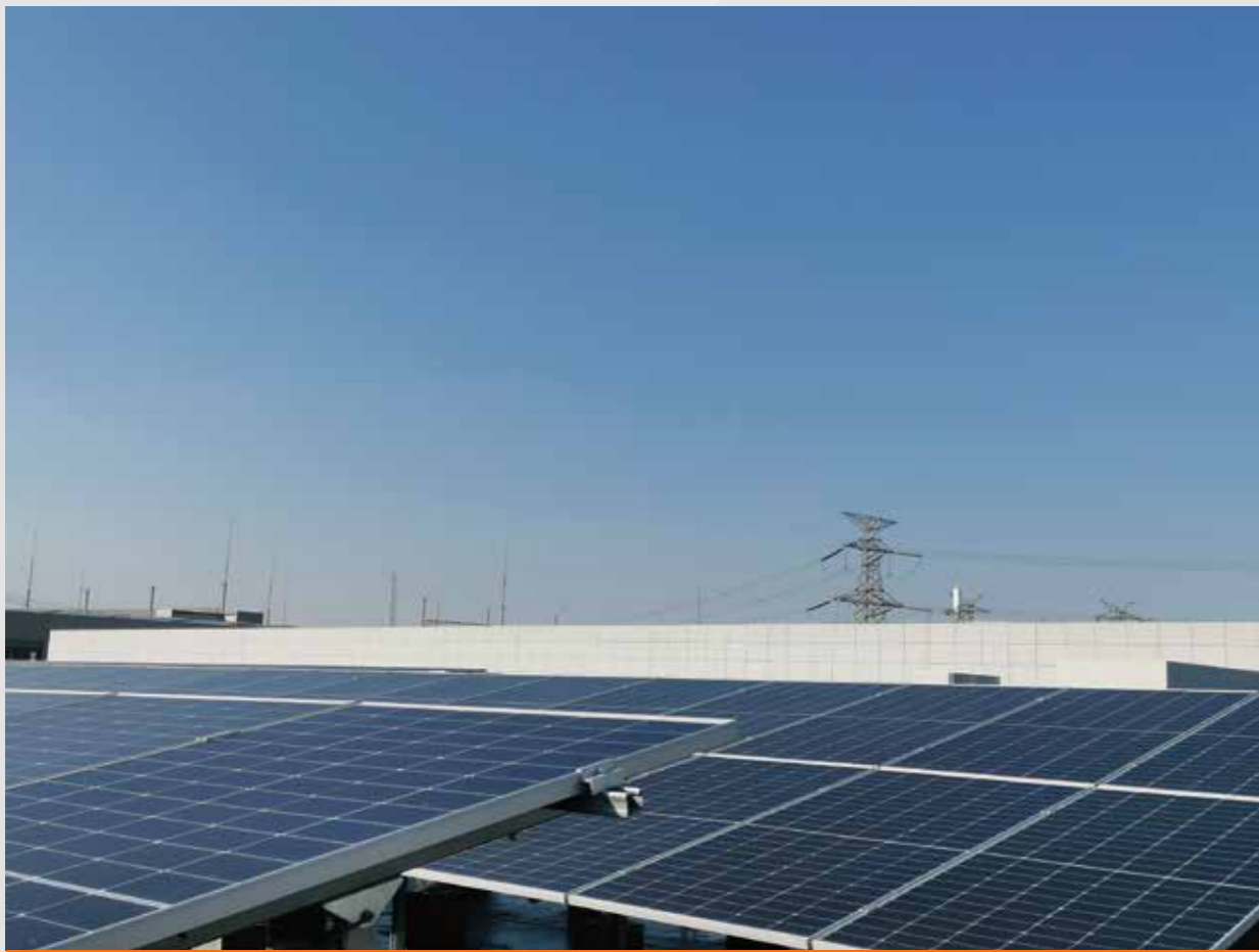
PV System on the Roof of the Company
